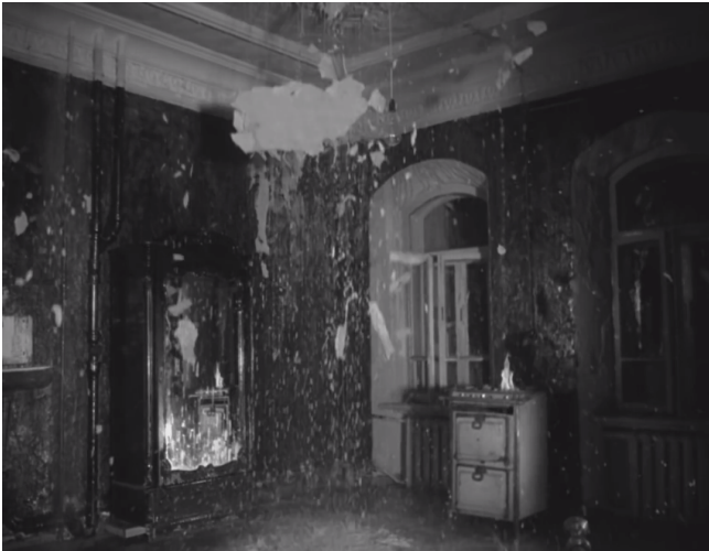
Figure 19: The decaying room as the ceiling plaster falls.
